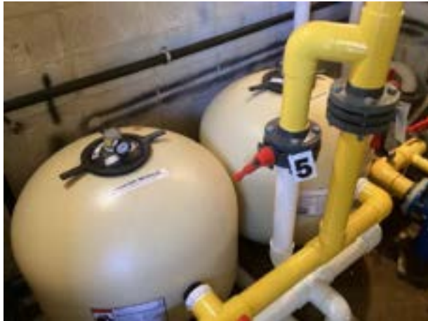
Pool mechanical equipment
