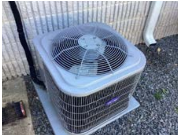
Split system condensing unit
