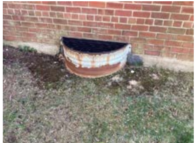
Window well- Note rust
