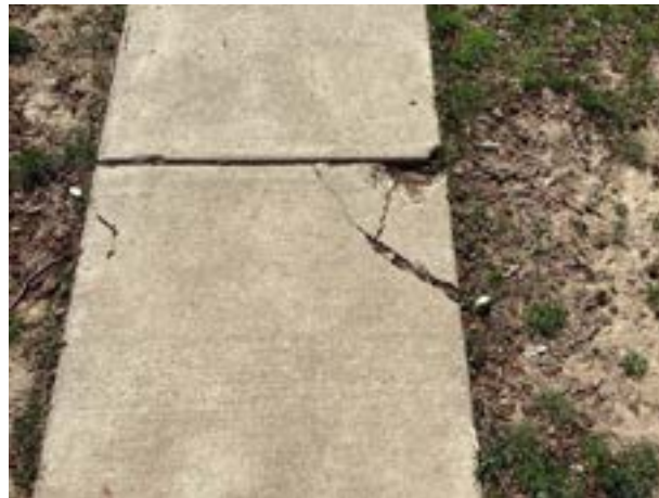
Sidewalk cracks and spalls
