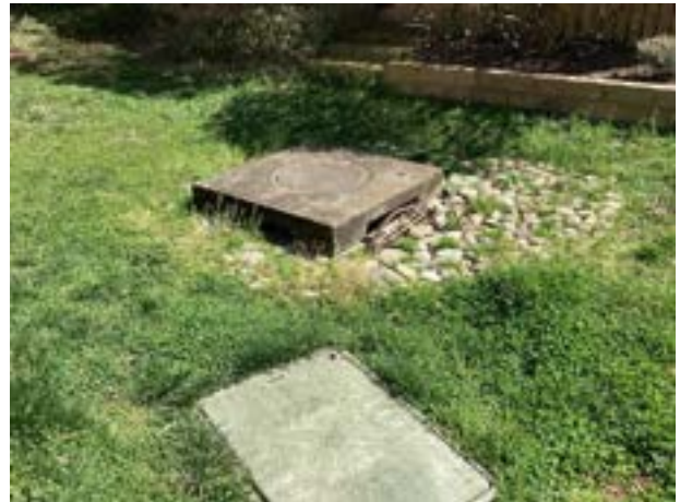
Landscape catch basin
