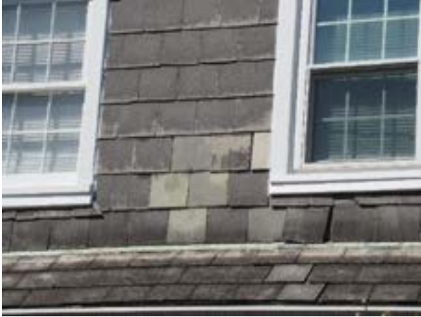
Previous repairs and shingle lift
