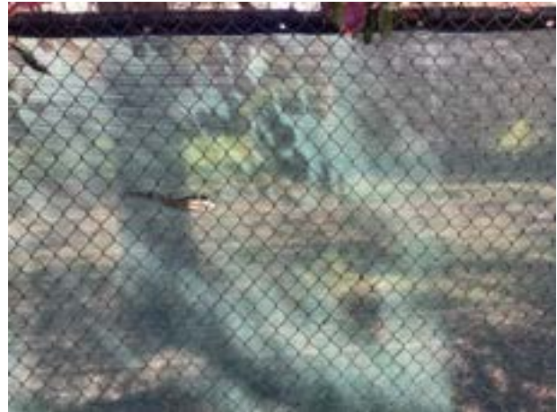
Chain link fence - Note fabric tear
