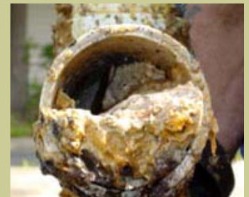
An Arlington County sewer pipe ruined by a FOG Clog.
