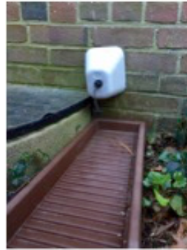
This spigot has been prepared for winter and has a low-cost Styrofoam hood affixed to it that provides additional protection from the harsh winter weather.
