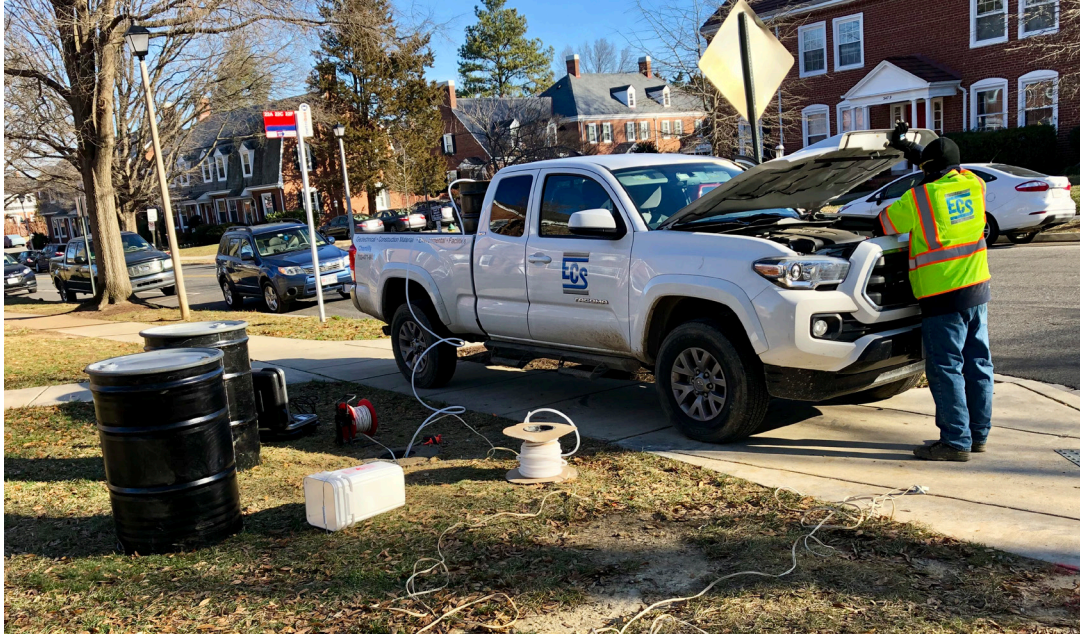
This photo shows the installation of the permanent test well at the corner of S. Stafford and S. 35th Streets.
