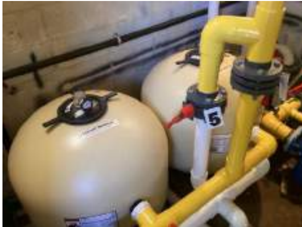
Pool mechanical equipment
