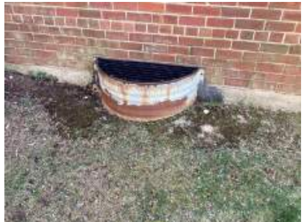
Window well- Note rust
