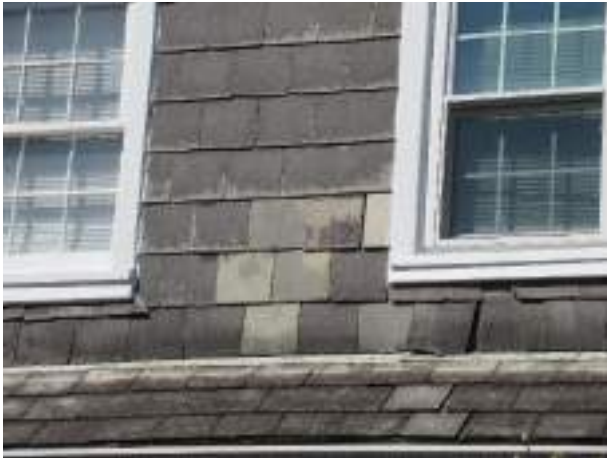
Previous repairs and shingle lift
