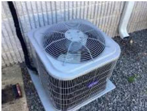
Split system condensing unit
