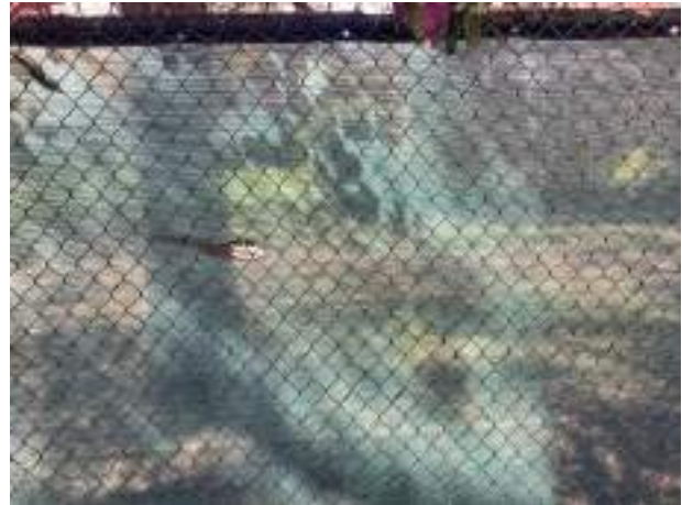
Chain link fence - Note fabric tear
