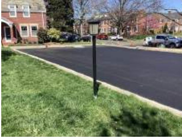
Light pole and fixture
