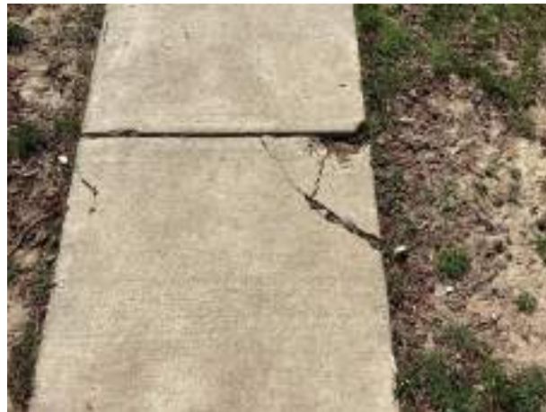
Sidewalk cracks and spalls
